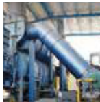
Waste to Energy
