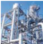
Waste Heat Recovery
