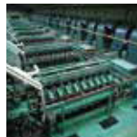
Power Plants & Multi Utility Plants
